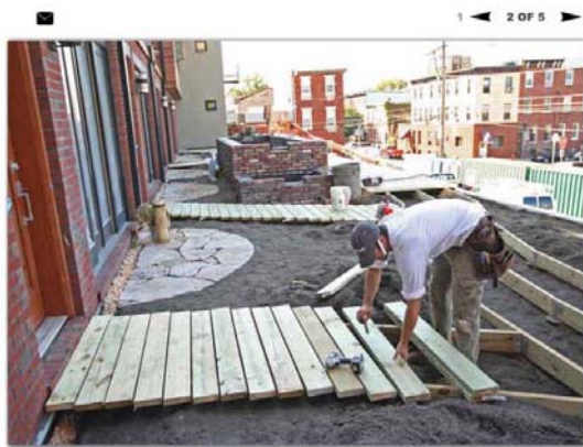
Mike Reagle builds a front walk at the condos. Bricks from the old Dooley's Icehouse on the site form a ice pond in the background.
